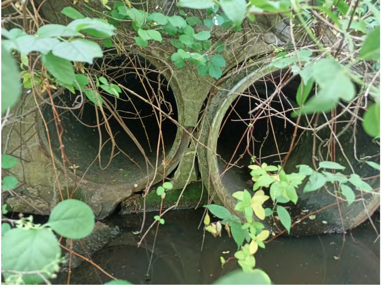
Outfall ID #D0204 (on right)
